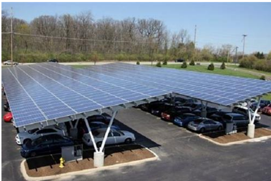
Figure 4-1. Example of a solar PV carport with steel support structure
