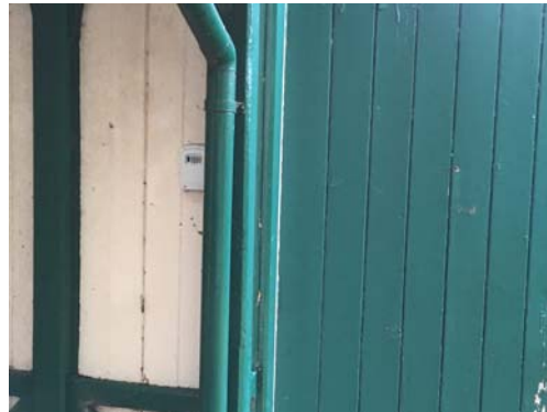
Picture 4 – key safe, left hand side of porch
