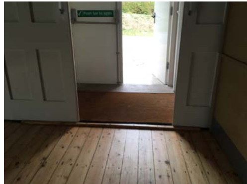
Picture 4 – Lip on access to/from main hall
